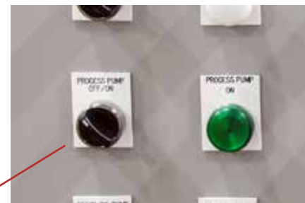
Typical Process Pump Switch on units with MZC control.
