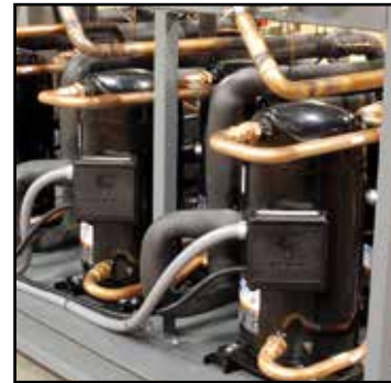
Compressors. Configuration may be different on specific units.
