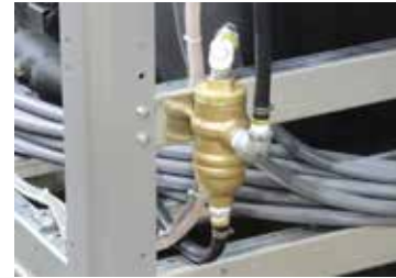
Typical water make-up level switch
