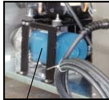
Electric motor Figure 3.2D
