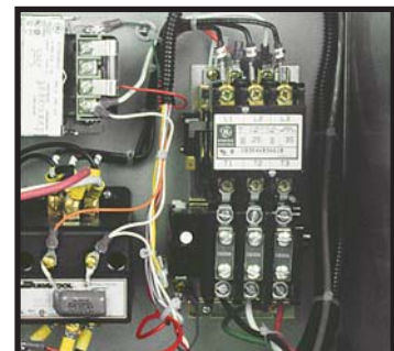
Motor overload relays and reset lever
