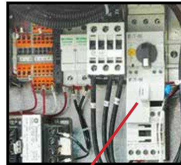
Pump Motor Control
