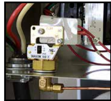
Panel mounted pressure switch
