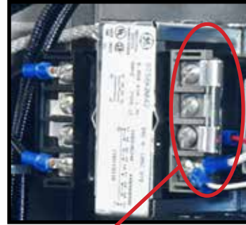
Control circuit transformer fuse
