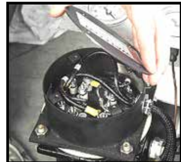
Heater junction wires
