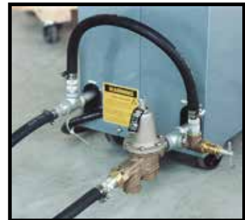
Typical pressure reducing valve installation (shown on S-925).
