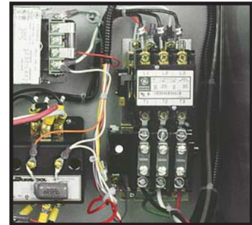
Motor overload relays and reset lever Figure 3.2D
