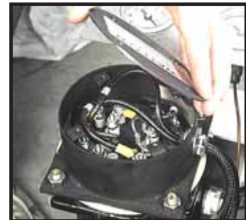
Heater junction wires
