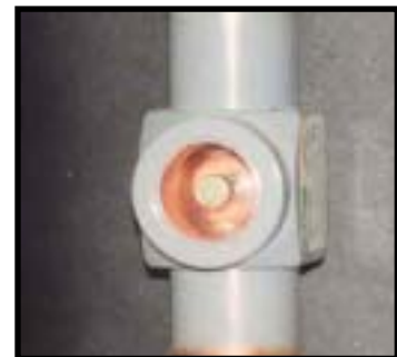
Refrigerant sight glass Figure 6.2D
