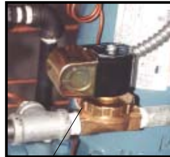
Typical water make-up solenoid valve
