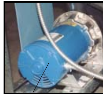
Pump motor Figure 5.5B
