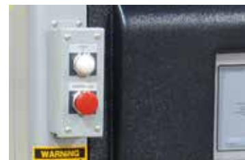
Emergency stop button. Shown with Power On light.
