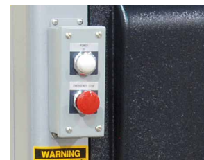
Emergency stop button. Shown with Power On light.
