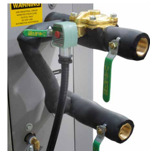
Typical overhead piping kit. Shown with optional process line shut off valves. Process line shut off valves are also shown in this photo.
