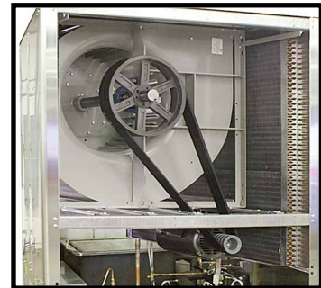
Typical blower assembly
