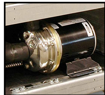
Pump motor Figure 5.5B
